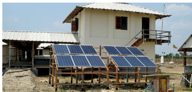
Power supply to a hospital
